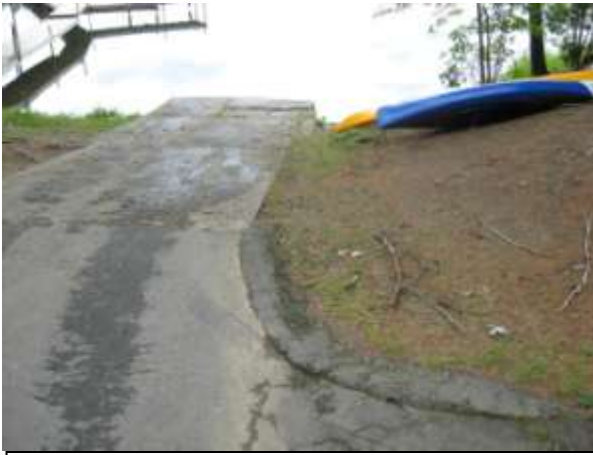
Boat ramp without any infiltration #8
